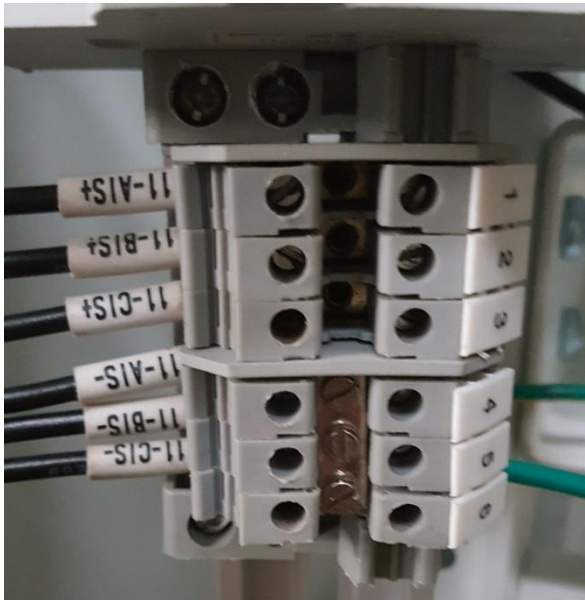
Figure 4-9 Rack-mounted APF External CT Terminals
